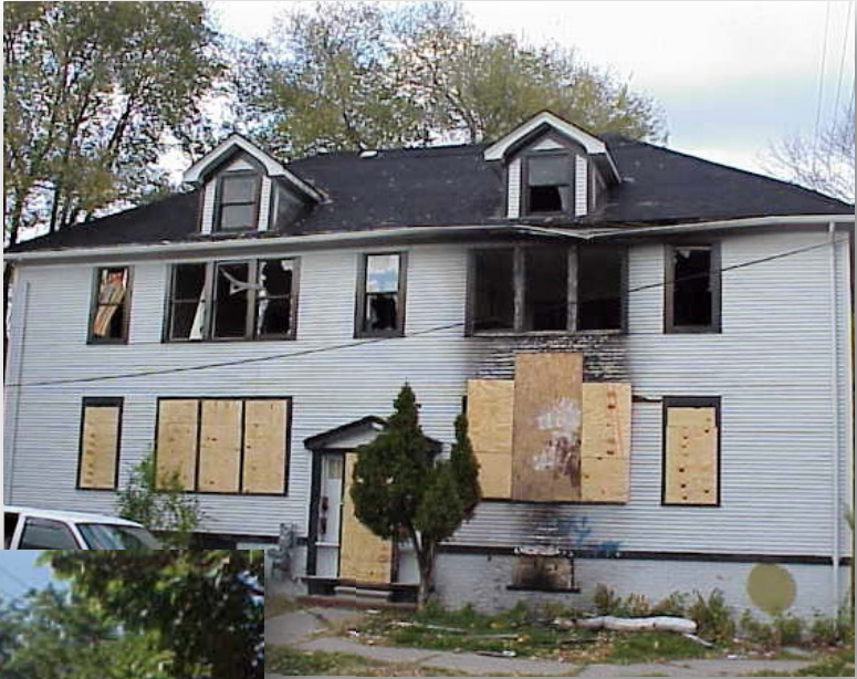
Fire damage... Detroit apartments before and after
